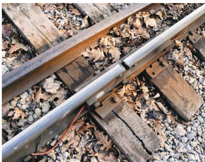
Figure 1.2 Without expansion gaps between the rails, the track would buckle in hot weather.
